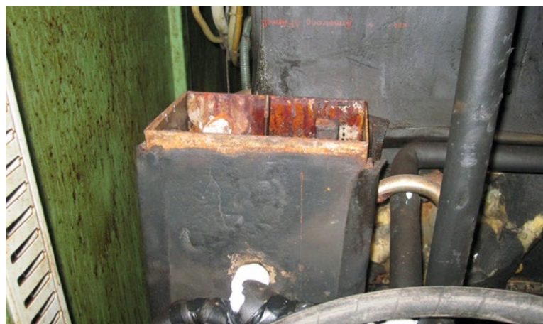
Picture 11: Machine parts corroded
