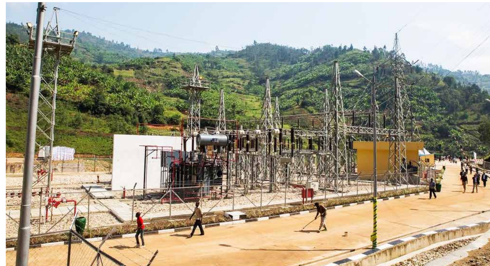
© Launch of Nyabarongo Hydropower Plant- Muhanga, Rwanda, 5 March 2015. Photo from the Office of the President
