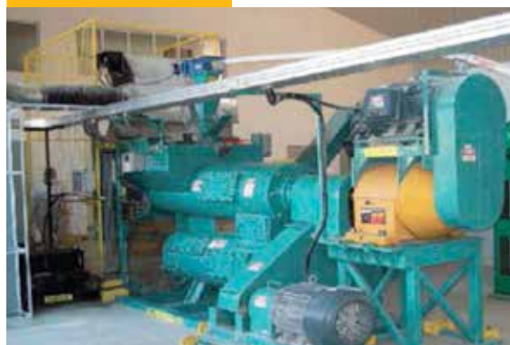
CHEMICAL DISINFECTION TREATMENT FACILITY FOR MEDICAL WASTE
